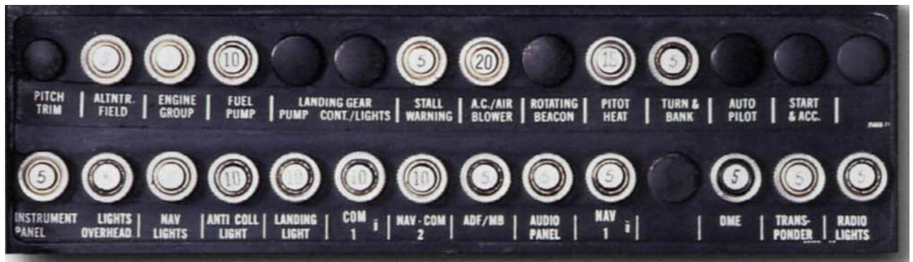
Figure 2-60. As a pilot, you should know the location of the circuit protection device for each electrical component. Normally, the component's name is printed on the circuit breaker panel near its associated fuse.
